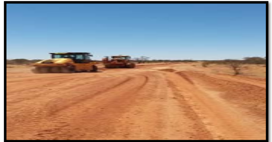
Flood Damage Mayneside Access
